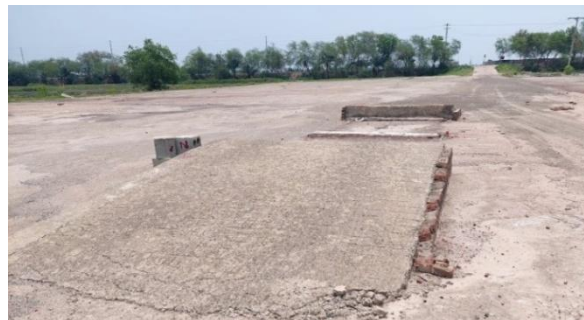
Figure 14: Pankhali yard no. 1, needs to be demolished (P-32)
