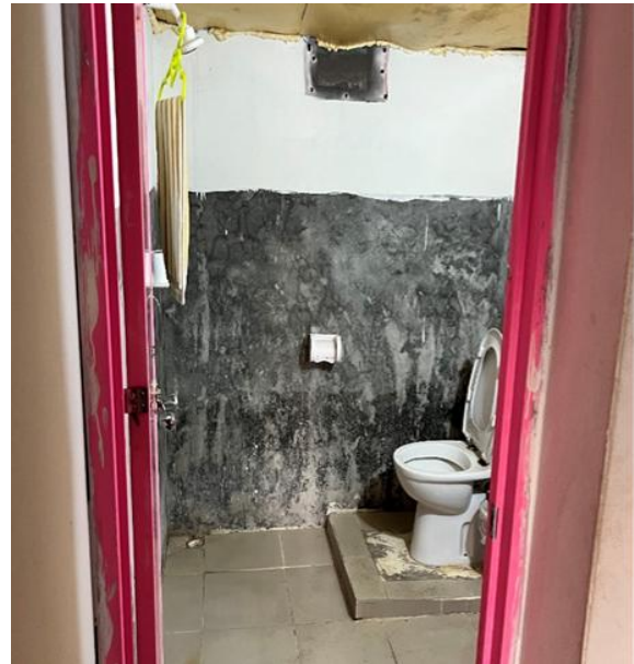
Figure 32: Toilet facility of Quarantine room of Polder 39/2C
